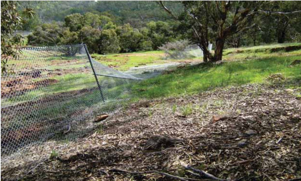
Figure 10 Fence Damage by Vandals at Site 4 During August 2013
